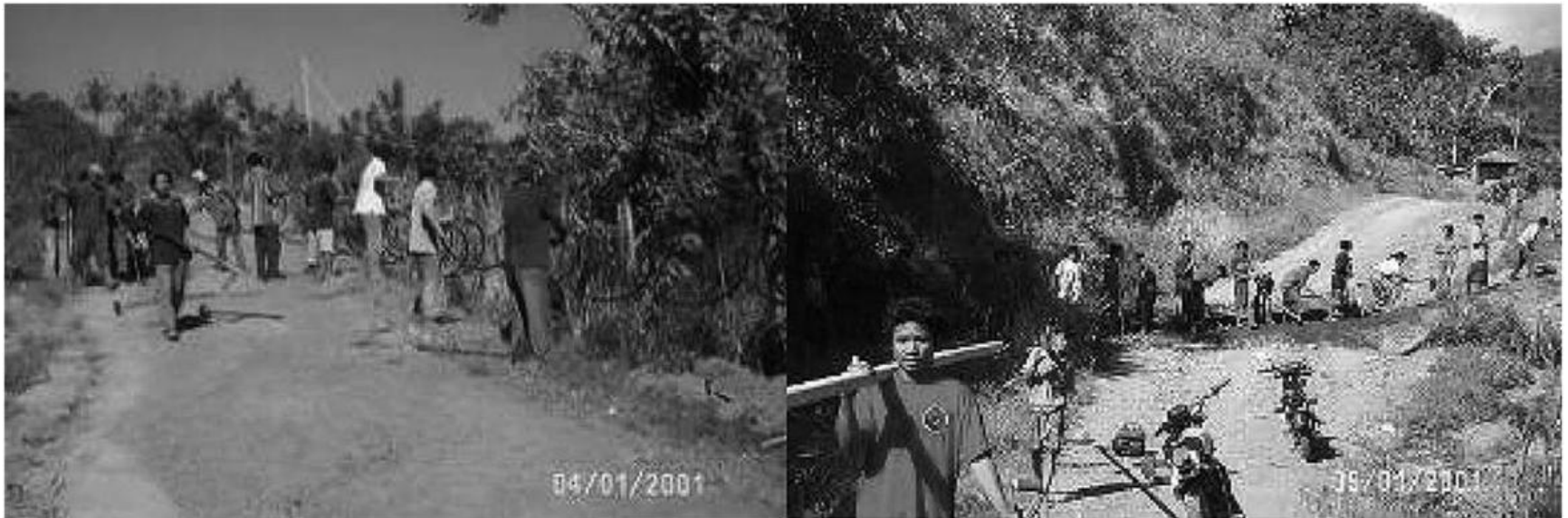
Figure 6. Pipe Laying Across Dirt Road for Supplying the Community Reservoirs from Mountain Spring
