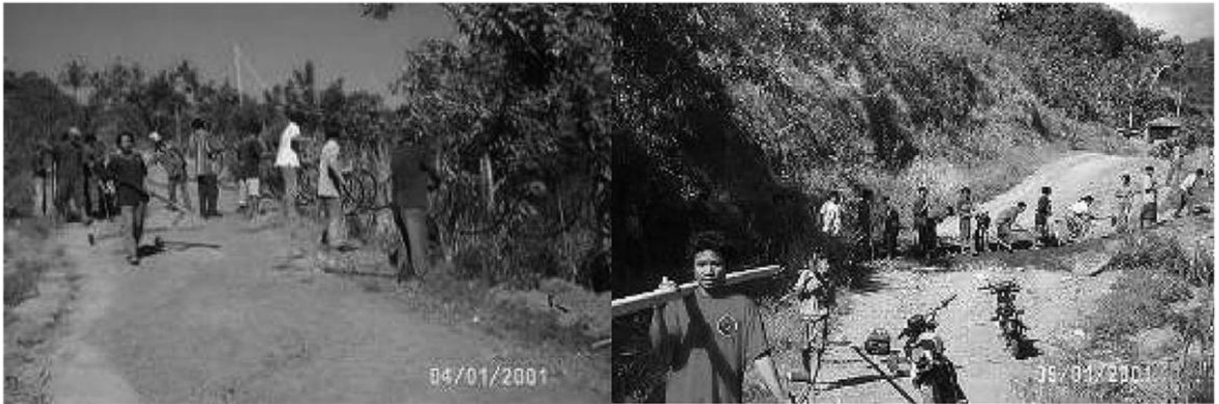
Figure 12. Pipe Laying Across Dirt Road for Supplying the Community Reservoirs from Mountain Spring
